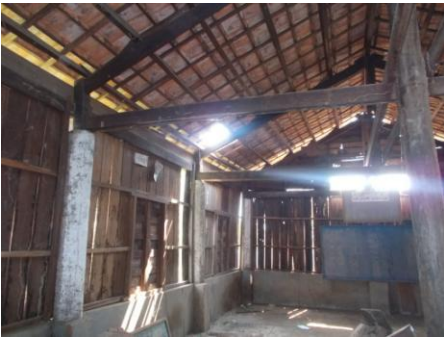
75 pre-school children and 65 primary school children did not have a good quality classroom. The original classroom had to be closed because it was unsafe.
